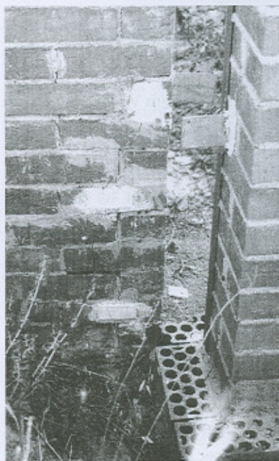
Figure 8. Corner of Long Brick Wall in Toledo. Figure 9. Crack at the corner of the same wall.
