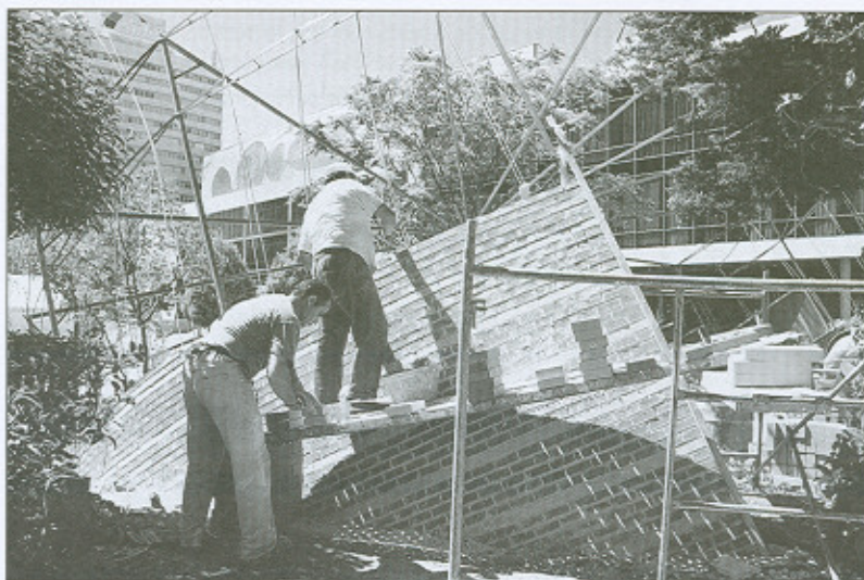
Figure 15. Left abutment under construction with sloping courses and seen from its internal convex face.
