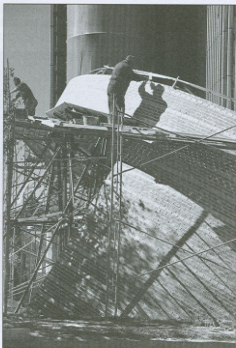
Figure 23. Oblique view of the arch centres supported on edges in the steel prop structure of the Arch, note the 5cm spacing between the arch centres and the struts that are filled by wedges.
