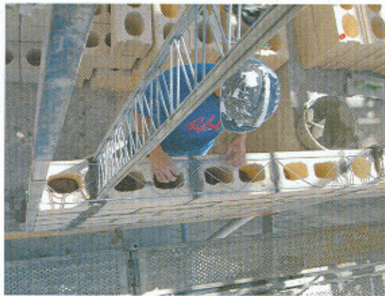
Fig. 15a Building of 7 m high straight panel enclosure walls with double reinforced ribs at the Hotel Marques de Riscal.
