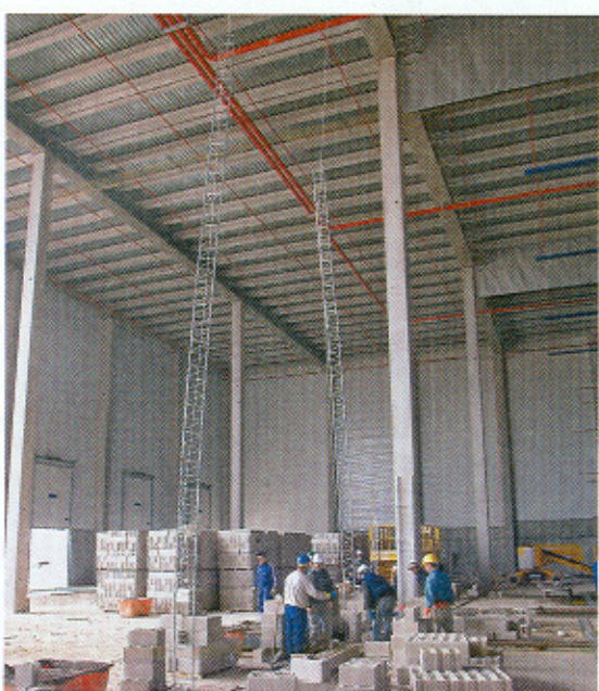
Fig. 13a Construction of a 15 m x 14 m double partition wall using the IMS.
