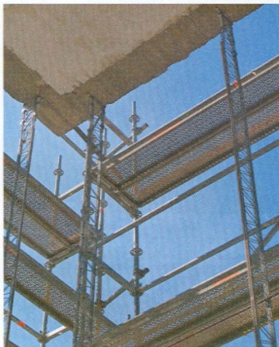
Fig. 14 Facing walls of the Hotel Marques de Riscal under construction. The walls are built in the IMS system with 7 m high double reinforced ribs.
