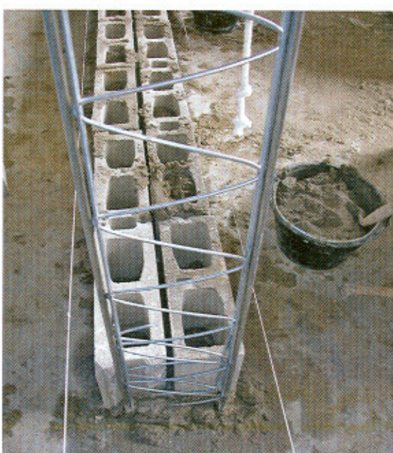
Fig. 13b Double wall with the rib tying both leaves of 15 cm hollow concrete block.
